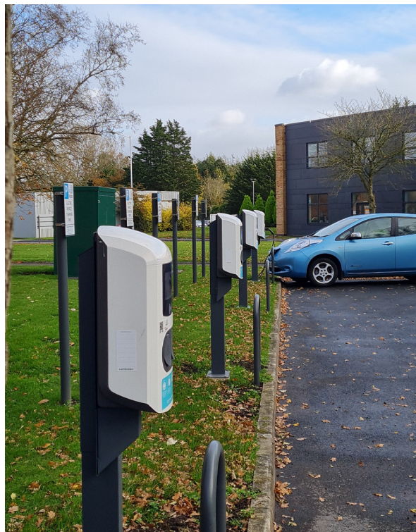
As part of our decarbonisation journey we have also installed EV chargepoints.
