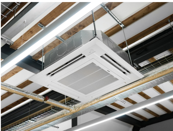
One of the ceiling units in situ.
