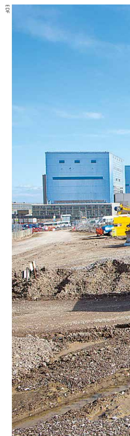
Work on the Hinkley Point C construction site with existing power stations in the background
